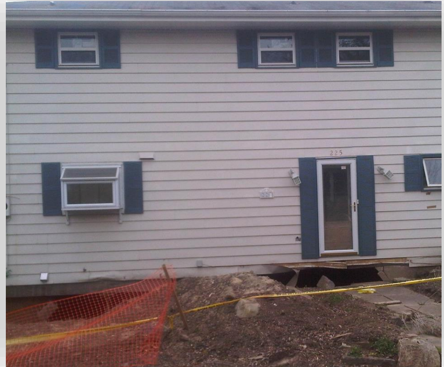
Foundation failure, West Pittston, PA (from FEMA Region III)
