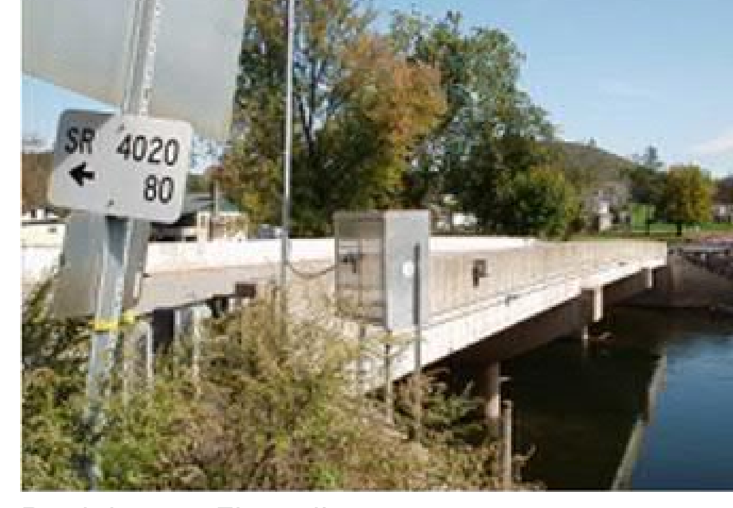
Problems: Flooding Mitigation Concepts: USGS Stream Gauge Reconstruction/Maintenance
