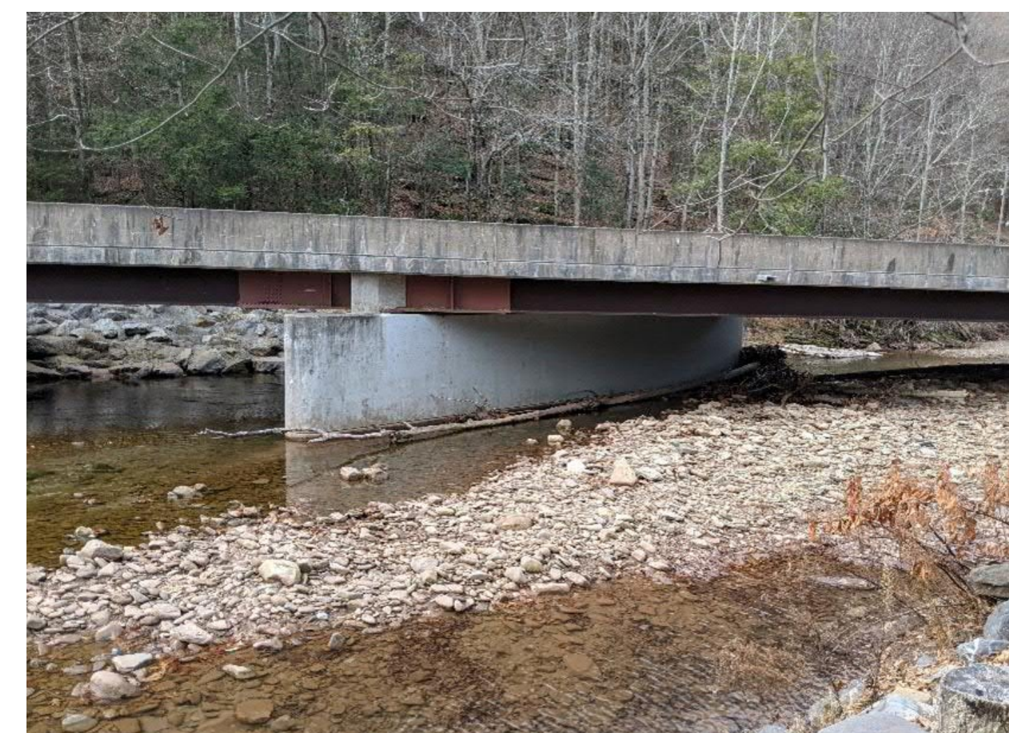
Problems: Flooding/Sedimentation Mitigation Concepts: Debris removal/ maintenance
