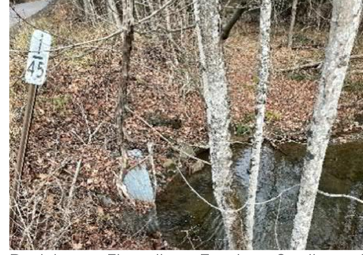
Problems: Flooding, Erosion, Sedimentation Mitigation Concepts: Culvert Replacement
