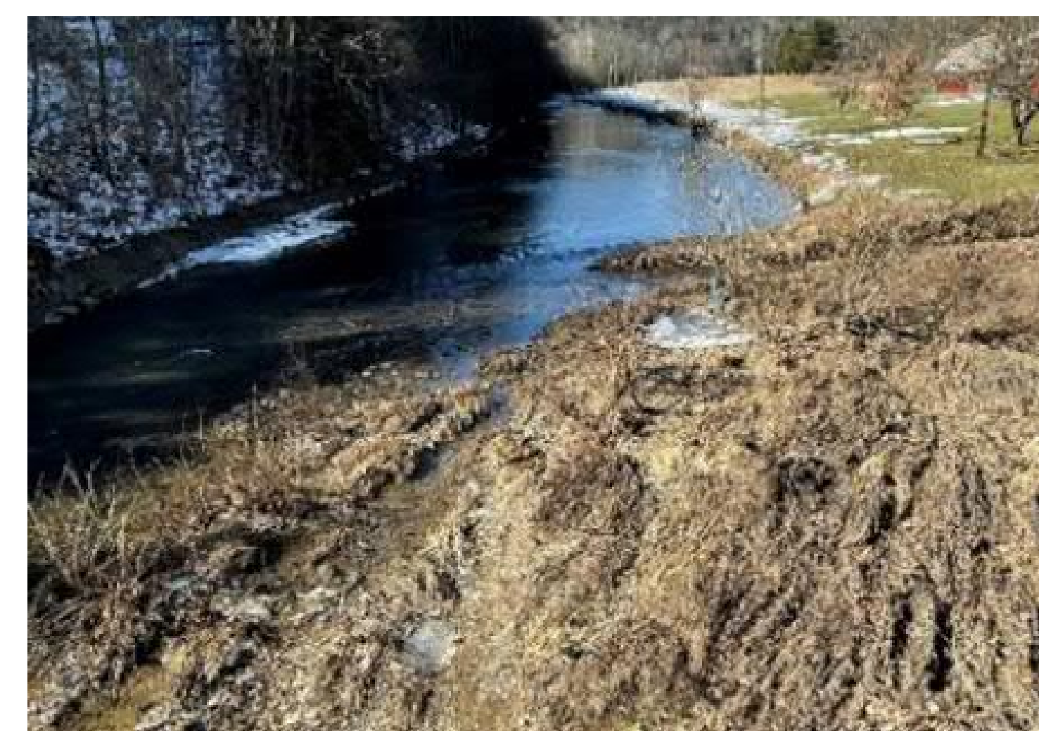
Problems: Sediment and Debris Buildup Mitigation Concepts: Sediment Removal
