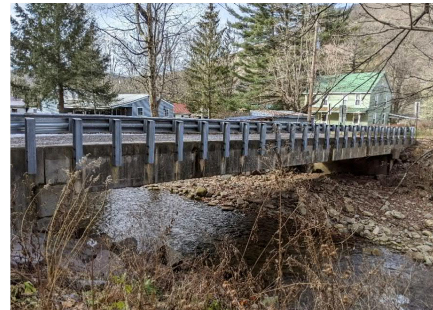
Problems: Flooding/Sedimentation Mitigation Concepts: Sediment Removal/Bridge Replacement
