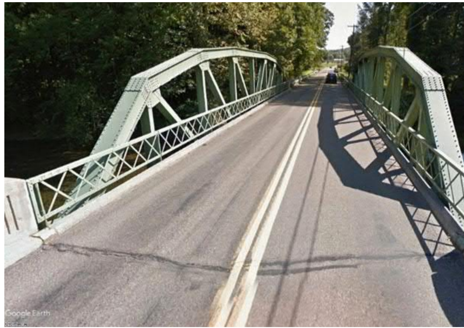
Problems: Flooding/Sedimentation Mitigation Concepts: Bridge Replacement/ Sediment Removal
